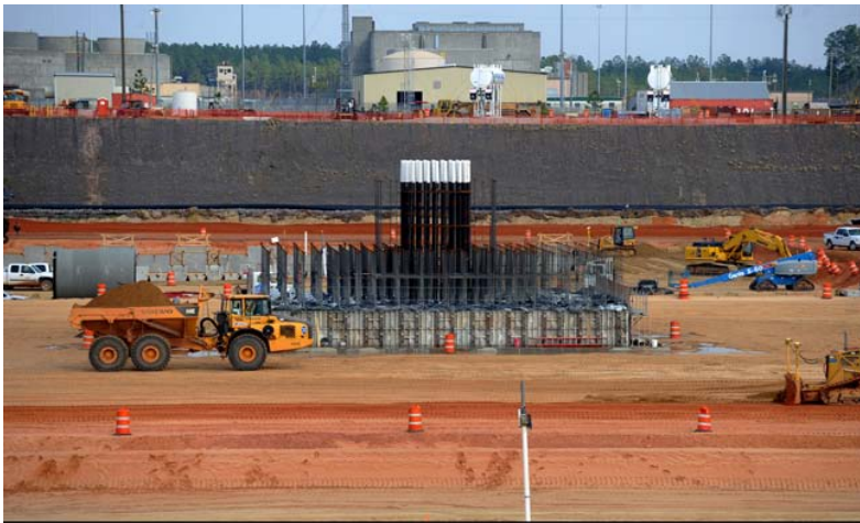
Construction of heavy lift derrick crane foundation and permanent counterweight, to be used to lift large components and modules into place for both Vogtle units 3 and 4. © Southern Company, Inc. All rights reserved March 14, 2011
