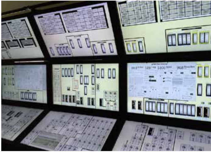
The COSS displays at the HSSL reflect the real-time plant parameters for normal and fault conditions. The display to the left is the operator interface panel and the display to the right is the plant systems overview.
