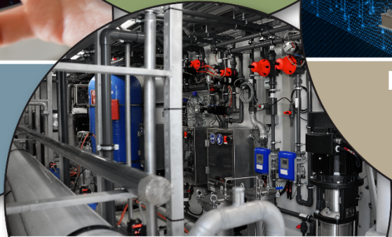
Advanced Control Systems
