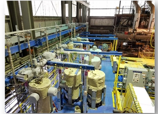
METL Facility , Argonne National Laboratory
